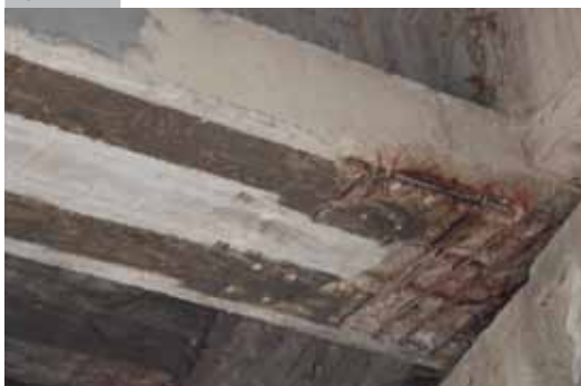
Drilling of the holes for plate anchoring and application of ARMOPRIMER 100 primer
