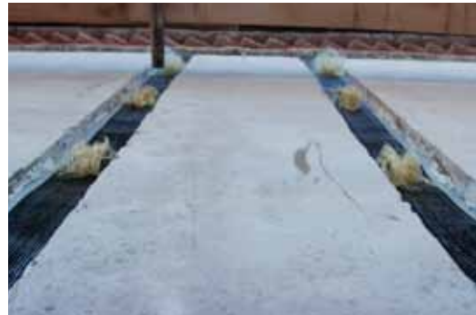
Laying of ARMOSHIELD C carbon fibre fabrics on the mortar housing grooves and insertion of ARMOGRIP connectors
