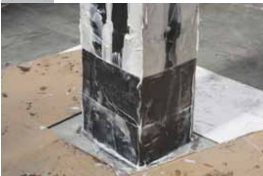
Laying of ARMOSHIELD C-SHEET unidirectional fabrics on ARMOFIX MTX resin and impregnation
