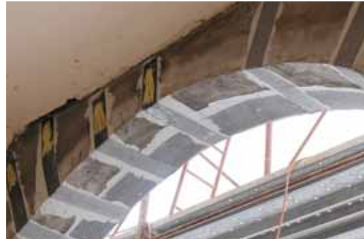
Application of ARMOSHIELD C-SHEET fabrics to the intrados and wrapping secured with ARMOGRIP connectors.
