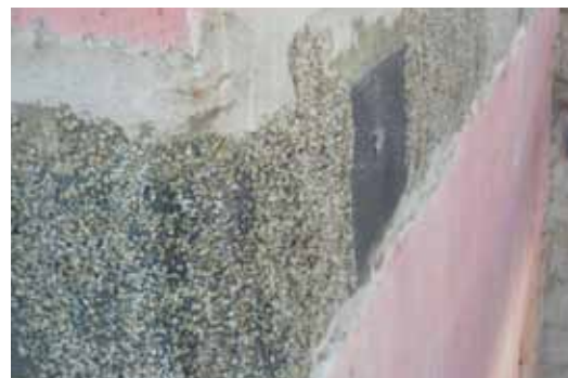
Detail of the final quartz sand sprinkle promoting the subsequent plaster application
