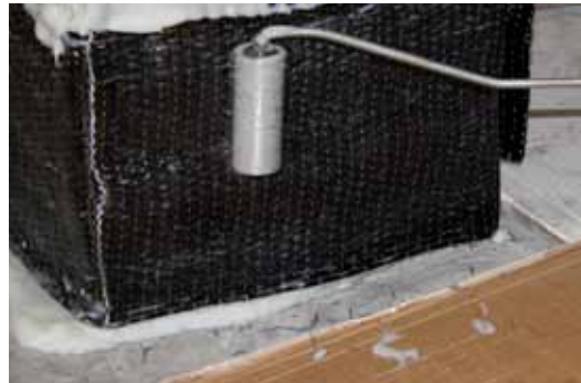
Laying of ARMOSHIELD C-SHEET fabric and impregnation with ARMOFIX MTX epoxy resin
