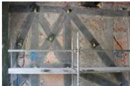
Wall reinforced on both sides with ARMOSHIELD C carbon fibre fabric placed according to the project model
