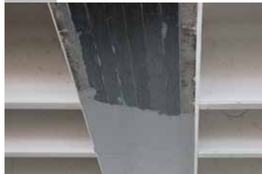
Apply ARMOFIX MTX adhesive over the plates until they are completely covered.
