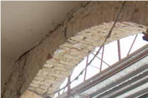
The arch before the intervention: complete removal of plaster or existing coatings
