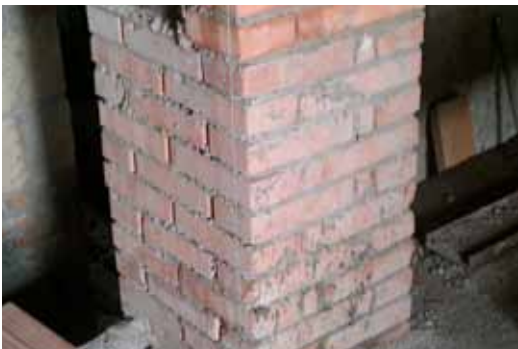
Compressed masonry pillar before intervention
