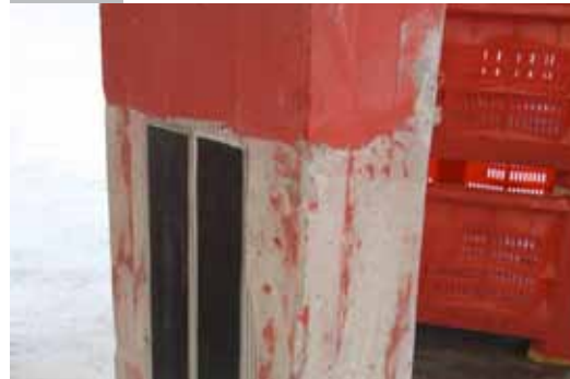
Application of ARMOFIX MTL epoxy adhesive for bonding and ARMOSHIELD CFK plates
