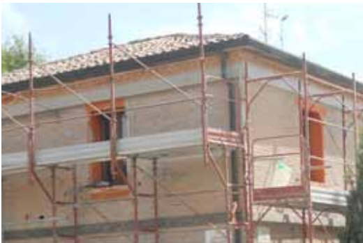
Overview of the intervention: wrapping performed at the top and at the floor slab
