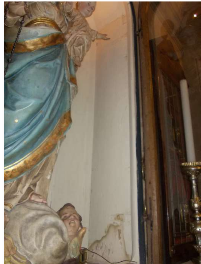
Evident rising damp
