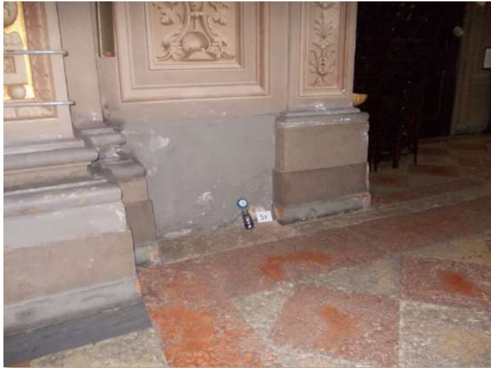
Deterioration of plaster with obvious rising damp
